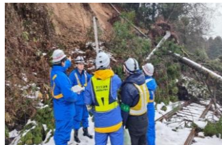
▲ TEC-FORCE damage assessment
